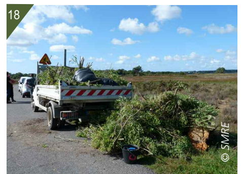
15. Groundsel bushes sprouting after uprooting. 16. 17. Uprooting of groundsel bushes using the telescopic tripod and chain hoist. 18. Removal of the waste to an incineration unit using a dump truck.
