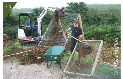
9. Storage in large bags for collection. 10. Uprooting, collection and storage of rhizomes. 11. Removal of the waste. 12. Scraping the surface with the small excavator. 13. Sieving the soil.
